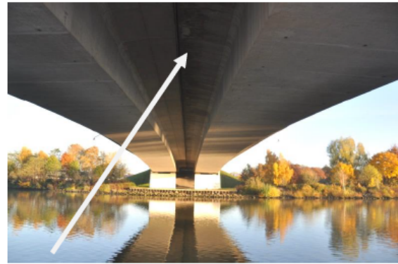
Figure 2. Location of the damaged cantilever (southern bridge).
