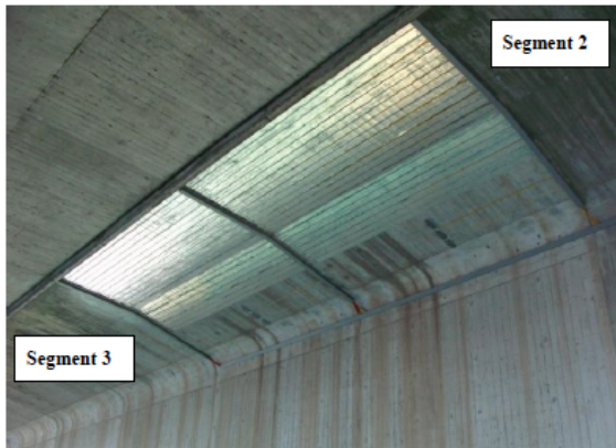
Figure 10. Test locations with the zinc anode material.
