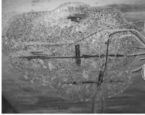
Figure 1. Spalled area of section 3.
